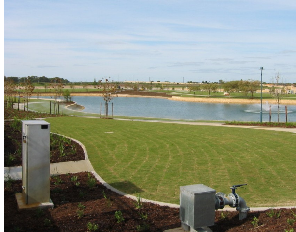
Local control panel with bore head
